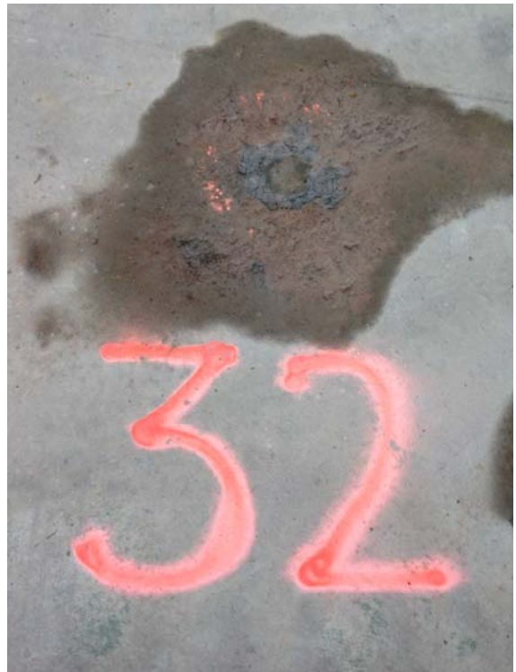
Boreholes are filled with a cement/bentonite mixture after they are completed. This is MHP-32 after grouting.
