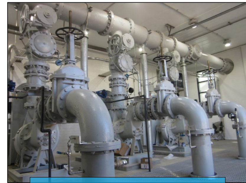
Surge Pump Station
