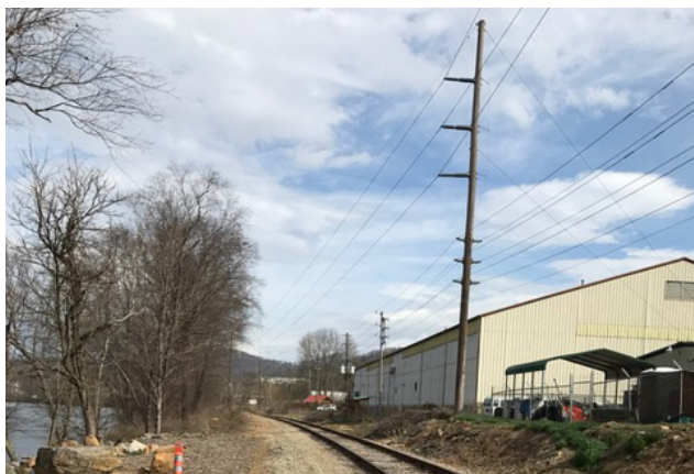
Overhead Transition Line Parallel to Railroad Line
