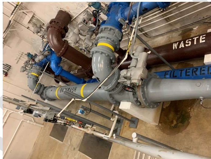
Figure 2-13 Media filter pipe gallery
