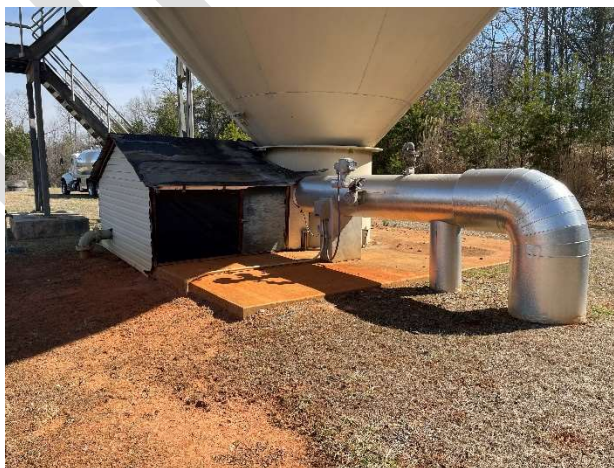
Figure 2-5. Influent and effluent piping at base of Claricone.
