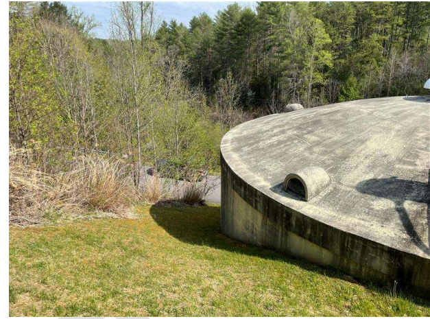
Figure 2-15 Top of clearwell facing north
