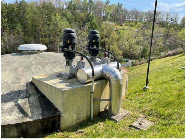
Figure 2-14 Finished water pumps
