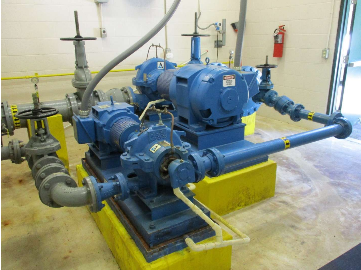
Figure 2-11 Surface wash (front) and backwash (back) pumps for media filters
