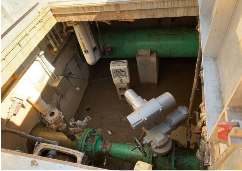
Figure 2-2. Chemical Injection Vault showing pipe from intake pump station (bottom) and 18 inch pipe from Claricone (top).
