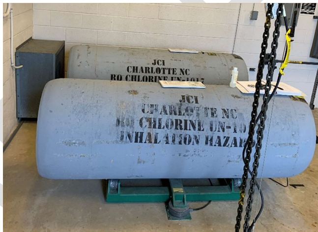
Figure 2-18 Chlorine gas tanks
