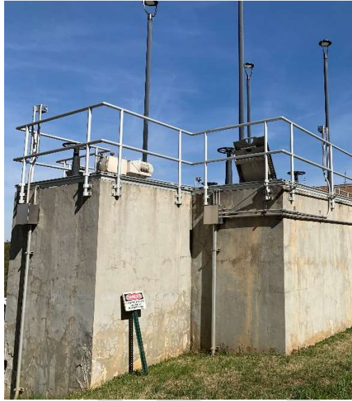
Figure 2-6. Flash mix tank exterior.
