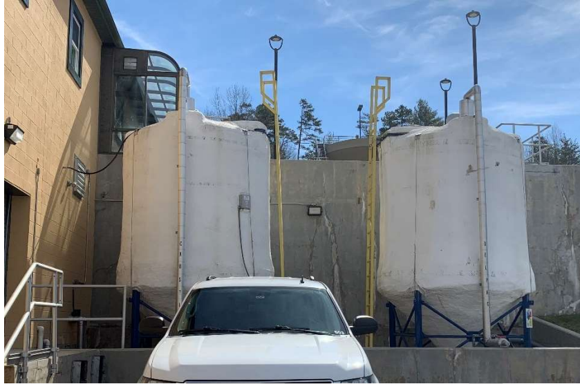
Figure 2-17 Alum (right) and caustic (left) bulk tanks
