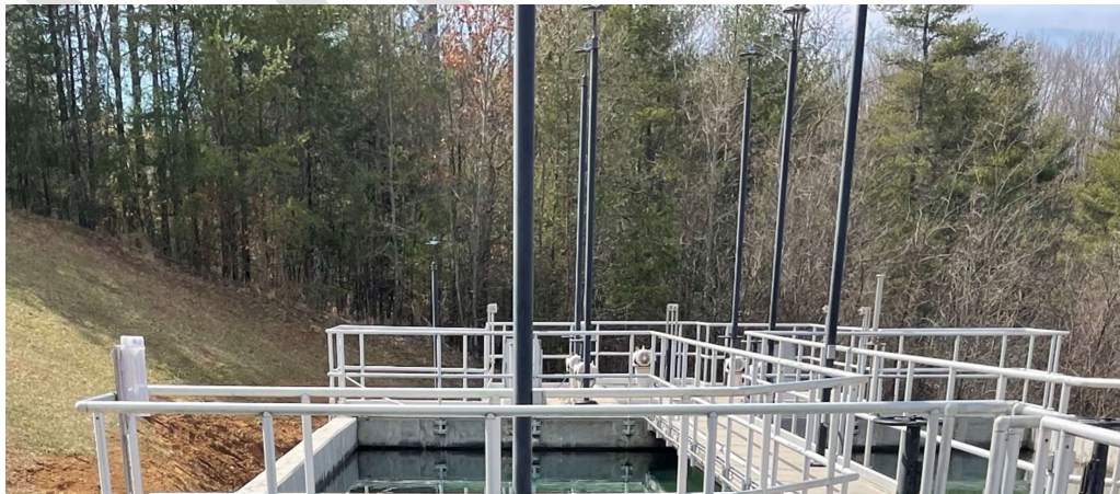
Figure 2-7. Top of flocculators looking west towards flash mix
