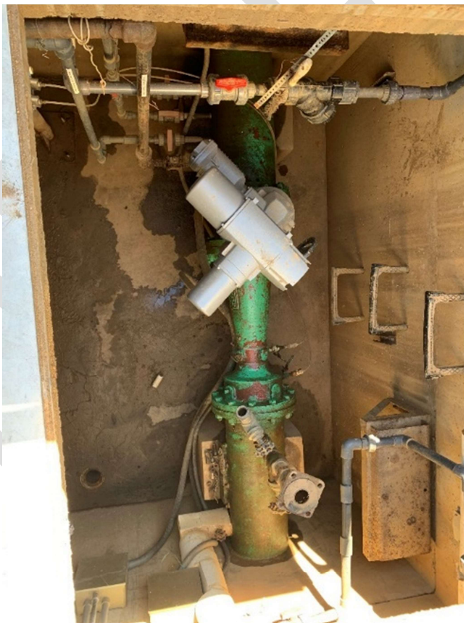
Figure 2-3. Motorized butterfly valve on 18-inch pipe from intake pump station.
